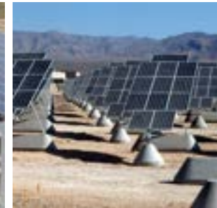
Solar farm, USA
